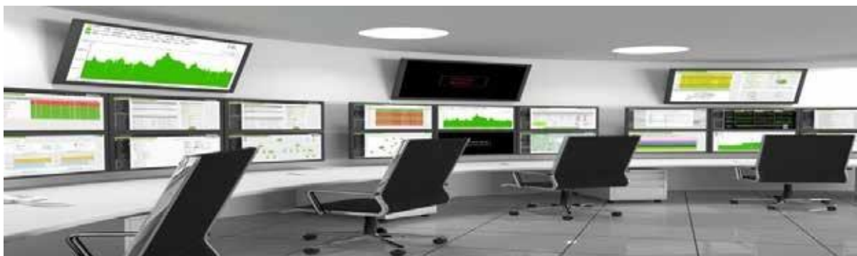
Figure 5-5: Smart meter operations centre
