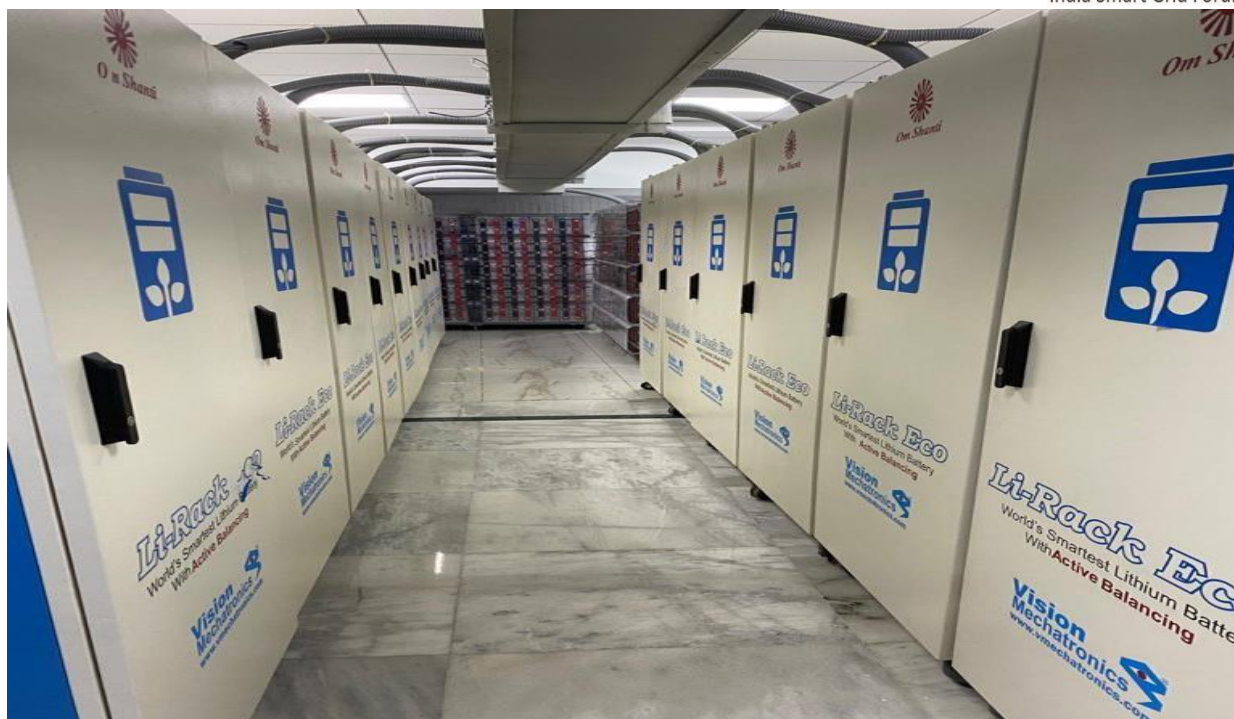
Figure 4: Mega Watt Scale Hybrid Energy Storage with Lithium-Ion Battery
