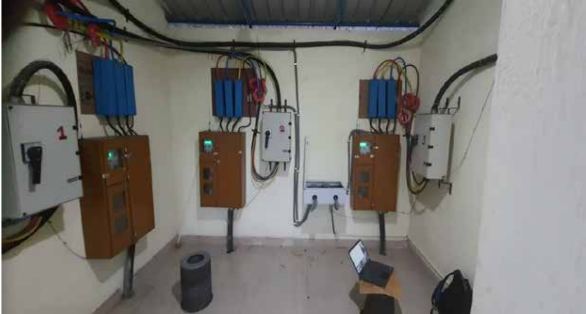
Figure 3-4: Meter room at Lake bus depot, Kolkata – PQM installed
