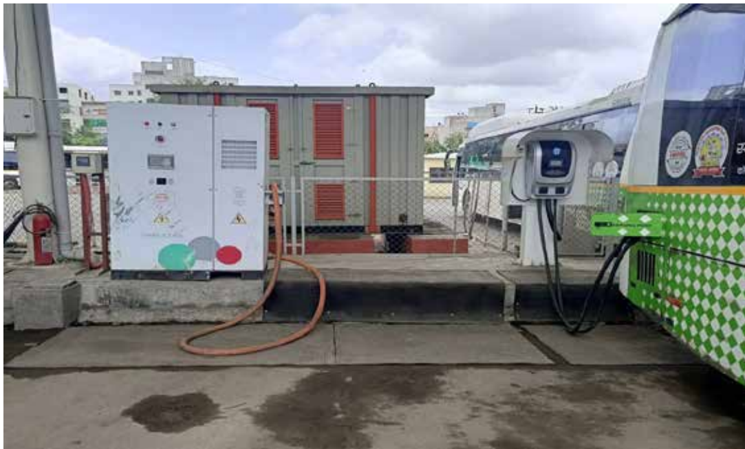
Figure 2-3: EVSE installed at PMPML Bhekrainagar bus depot, Pune
