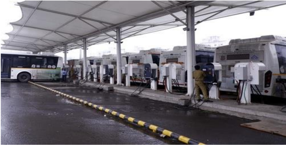
Figure 2-2: Chargers installed at PMPML Bhekrainagar bus depot, Pune
