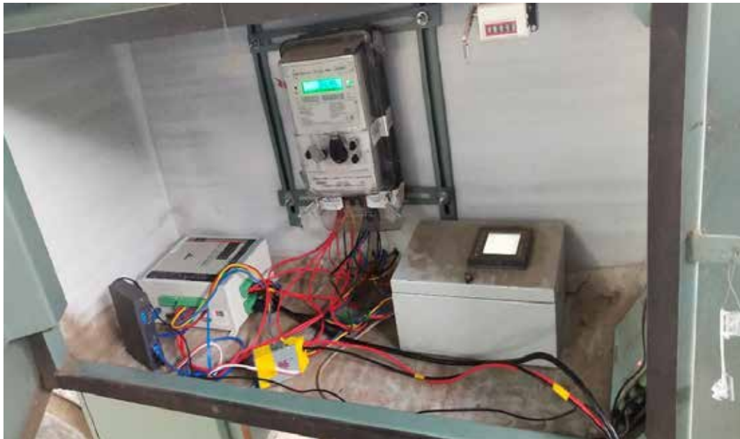
Figure 2-7: Installed PQ meter at 22 kV substation
